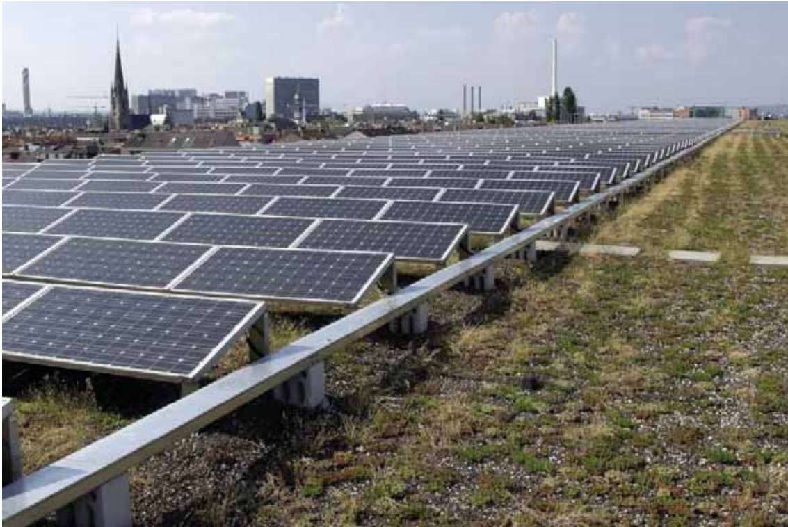
Messe Basel | Photovoltaikanlage
