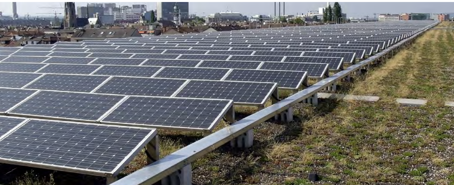
Photovoltaic system on the roof of Messe Basel
